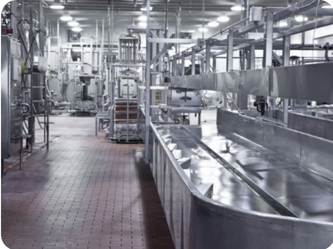
Cleaning and disinfection is important in the production environment in beverage processing
