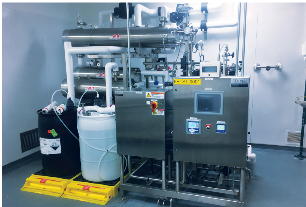
A HTST mid-scale unit operation
